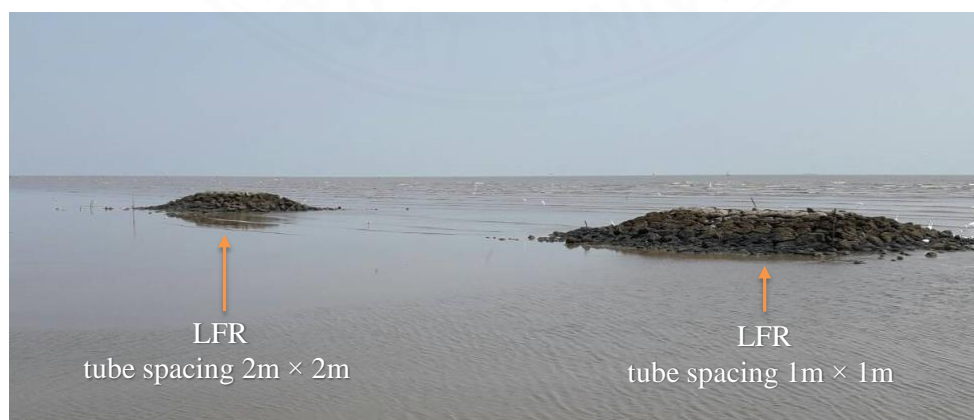
Figure 1.5 Test embankments of this study with 1\text{m} \times 1\text{m} and 2\text{m} \times 2\text{m} LFR systems
