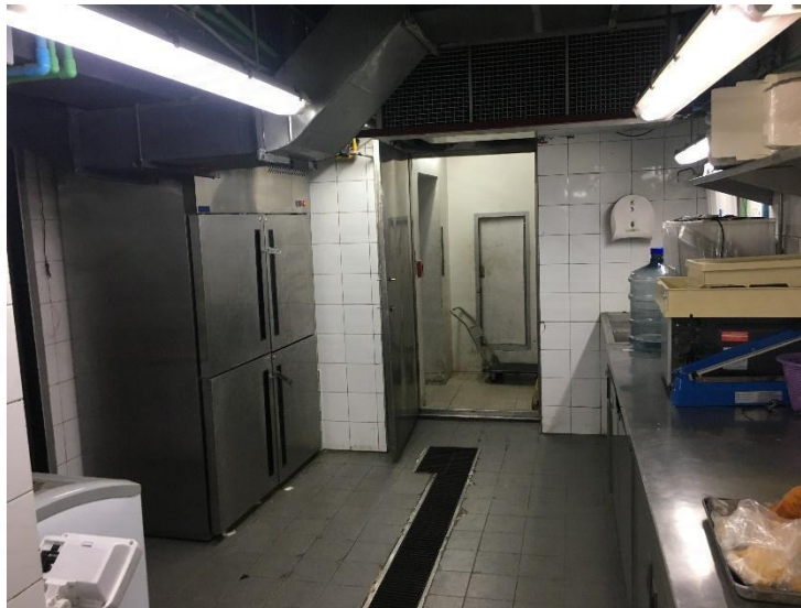
Figure 4.18 Floor Drains to Keep Water Out of the Flooring, with Some Worn Out Tiles
