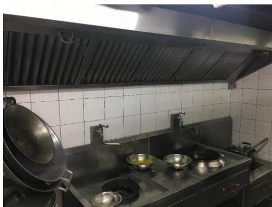
Figure 4.16 Ventilation Hoods Over Cooking Areas
