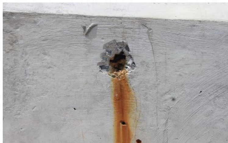
Figure 1.3 A reinforced concrete beam in a water retaining wall with iron sulfide deterioration showing pop-out of concrete (Saengsoy et al., 2021)
