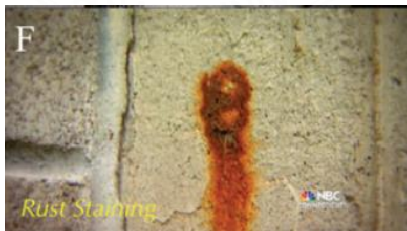
Figure 1.1 A reinforced concrete beam in a water retaining wall with iron sulfide deterioration showing rust staining on the concrete surface (Jana, 2018)
