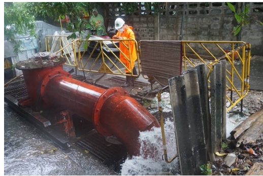
(b) Drainage Pipe
